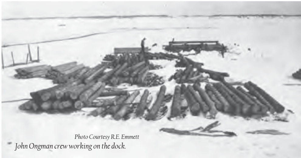
Photo Courtesy R.E. Emmett John Ongman crew working on the dock foundations in winter of 1920-21.
